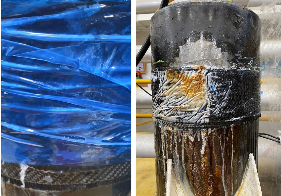
Figure 11.—Photographs of Product E at the end of the Weeping Trials. Left: water seeping underneath the compression film. Right: Corrosion product visible within the Product E repair.
