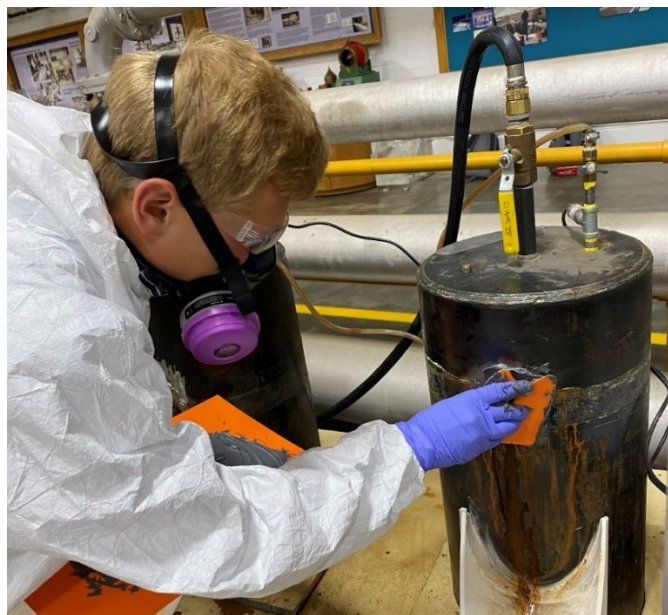
Figure 6.—Research team member applying an epoxy repair to the pressure vessel utilizing appropriate PPE.
