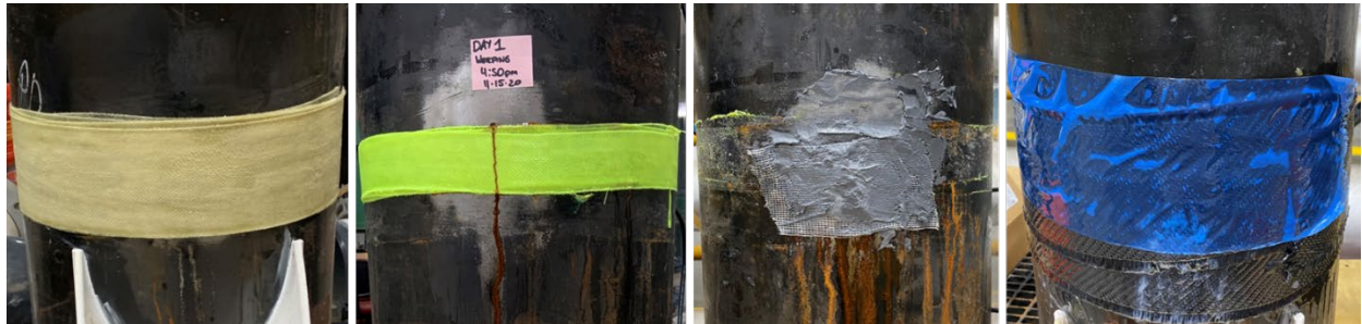
Figure 5.—Photographs of tested repair products. From left to right: Product A, B, C/D (visually identical), and E, as listed in Table 2. Note that Product E is mid-application in this photo with only one piece of blue compression film wrapped around, leaving the underlying composite repair visible at the bottom.
