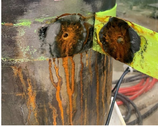
Figure 15.—Removal of repair Product B after Spraying Trial showing extensive corrosion underneath the repair.
