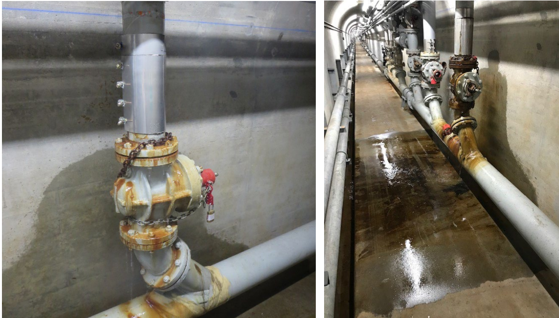
Figure 19.—Leak on 16-inch unwatering pipeline.
