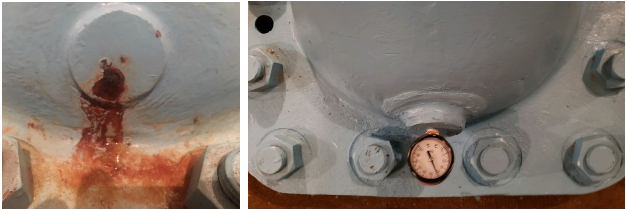
Figure 18.—Left: Photograph of pinhole leak in gate bonnet cover prior to repair. Right: Photograph of bonnet after repair showing the pressure gage and repair cap installed on the gate bonnet cover.
