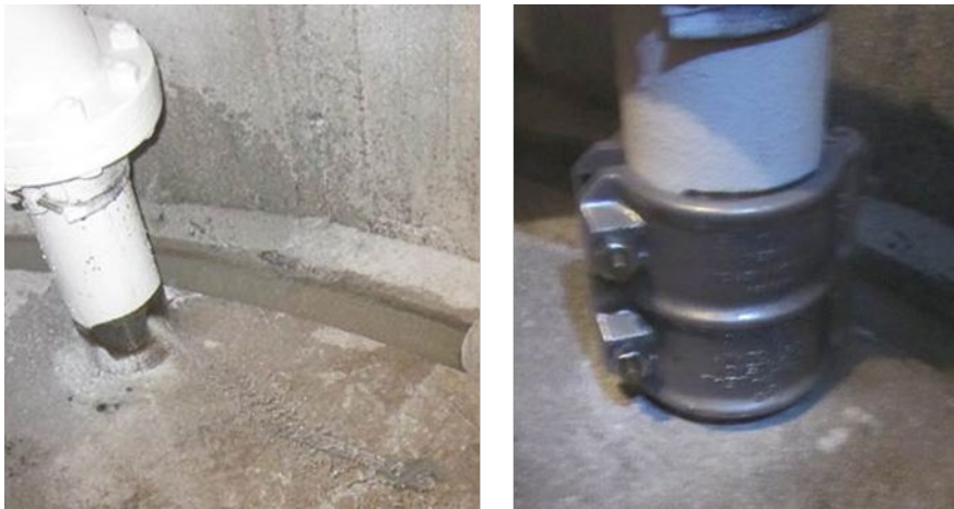
Figure 20.—Left: photograph of leaking pressurized pipe at a field partner facility. Right: photograph of the temporary clamp repair immediately after installation.
