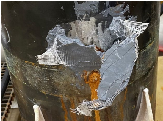
Figure 16.—Removal of repair Product C after Spraying Trial showing corrosion streaking the pressure vessel exterior where water continued to leak from the repair.
