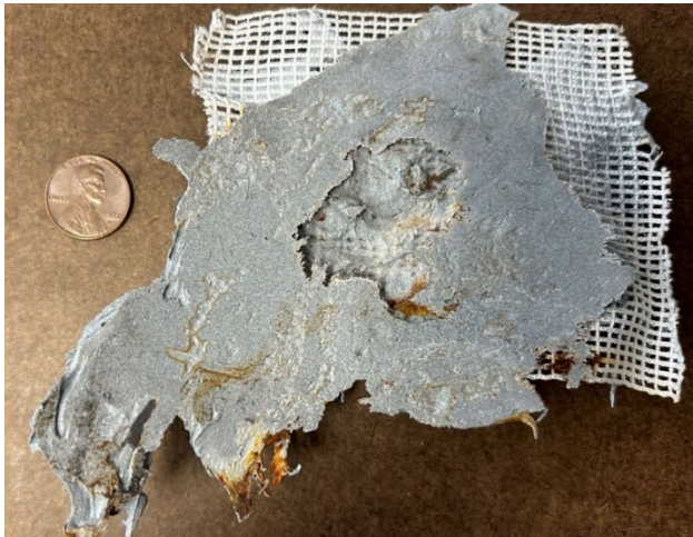
Figure 13.—Void in Product D repair material around the plug where leaking water prevented the material from curing properly.
